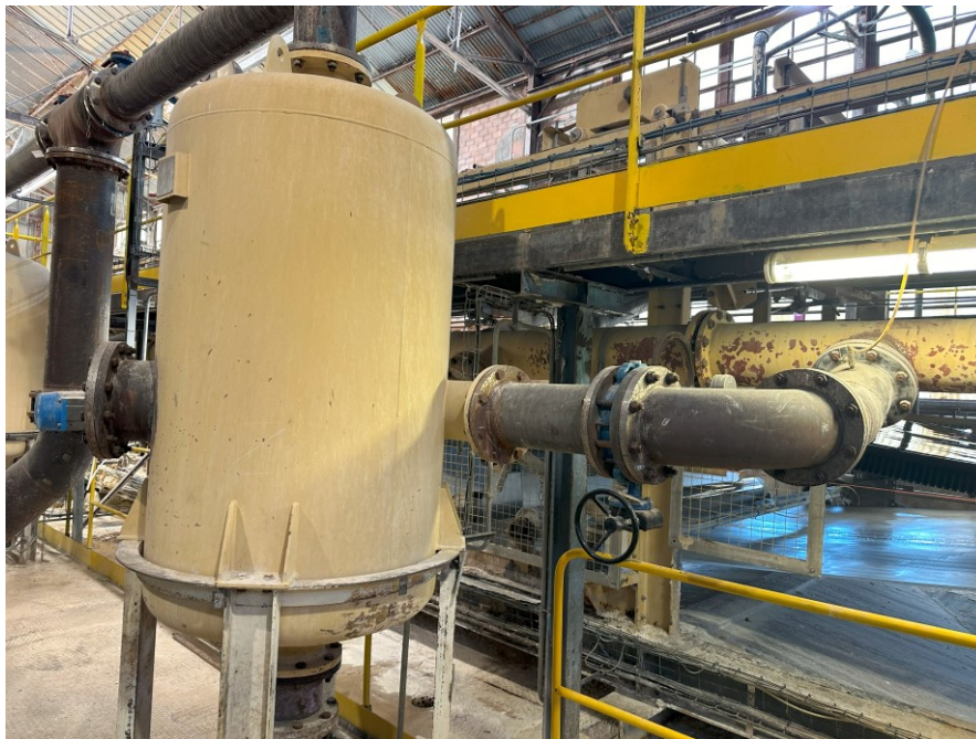
Figure 6. Rotated BA104 with the new F18 vacuum header tie-in point and a new flange with an instrument to detect high liquid levels (on left); new additional vacuum header just behind BA104.
