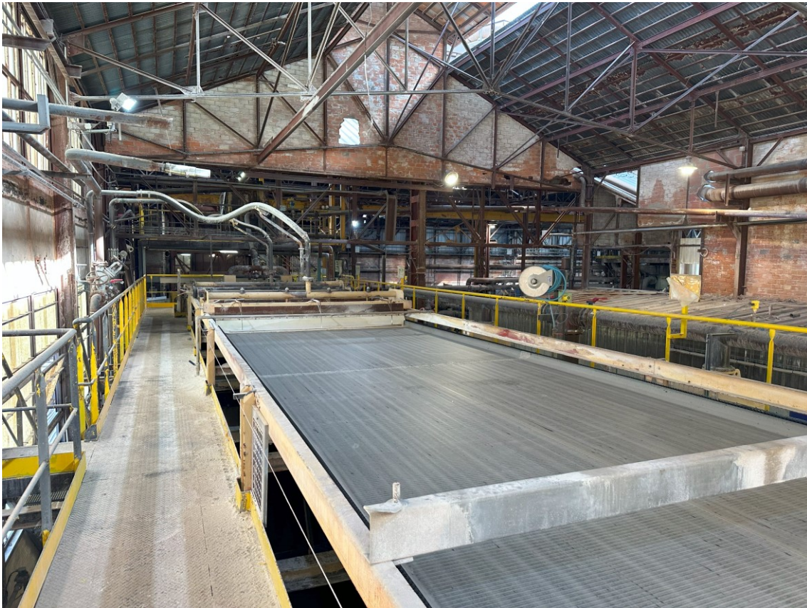
Figure 7. Belt Filter F18 showing the significantly reduced deliquoring and dewatering areas and the significantly increased drying area.
