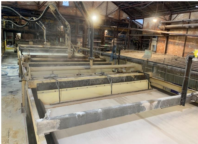
Figure 2. Belt filter F18 showing one of the weirs that limits the spread of wash water in the foreground.
